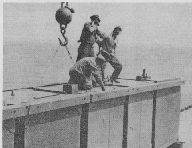
Fig. I-4 Pontoons being jacked at the top to allow the top assembly angles to fall into place.
